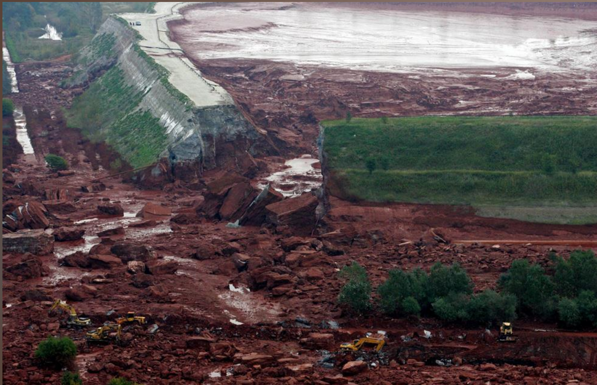
Ruptured wall of red sludge reservoir
